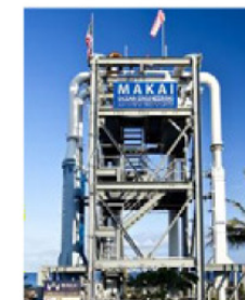
2015 : 100kW OTEC plant Grid-connected (NELHA/MOE)
