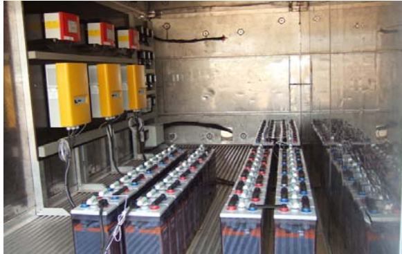
Battery station in Ghana
